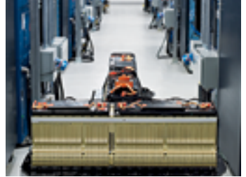
Uncovered look at the 288-cell lithium-ion battery pack.
